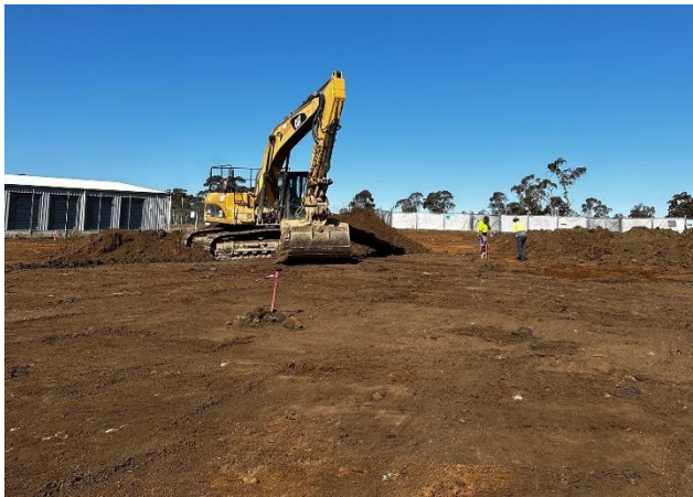
Site has been cleared of grass, levelled (cut and fill) and the set-out has been completed.
